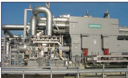
Figure 3: A motor-driven compressor is fitted with magnetic bearings in natural gas pipeline service in northern Holland. The power rating of the system is 23 MW and total rotor weight is about 11 tons
